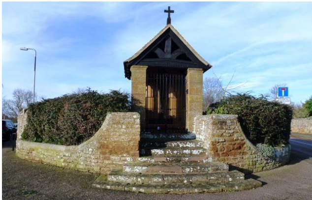
The war memorial. An example of a structure which is not listed but should be assessed for inclusion on a local list of heritage assets.
